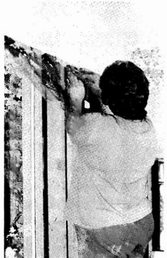
The kitchen will never be the same especially after Mrs. Dorothy Morales finishes with cutting away the old wire mesh that held up the plaster. This was taken in 1977.
